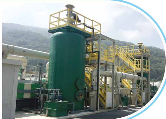
生物滴濾塔 Biotrickling filters
