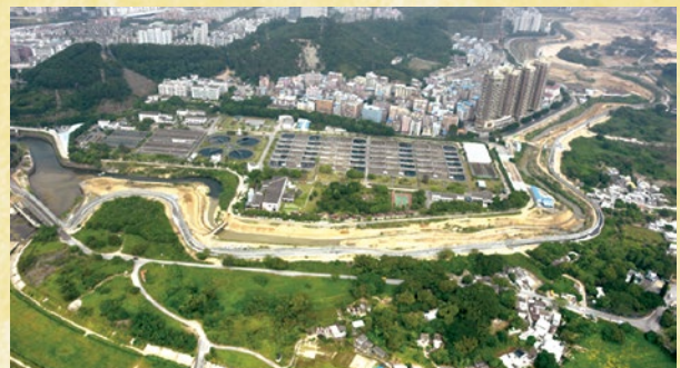
治理深圳河第4期工程的鳥瞰圖 Bird's-eye view of Shenzhen River Regulation Project Stage IV
