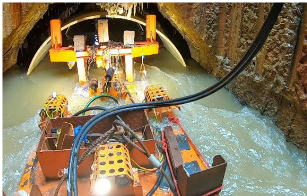
Deploying Robotic Machine for Lining Installation Works in the Existing Box Culvert with Live Sewage Flow
