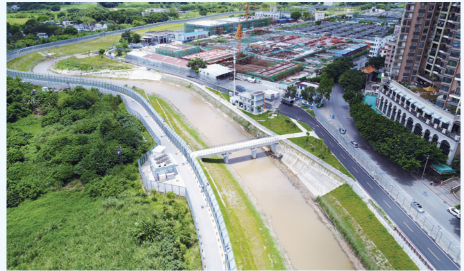
The Stage 4 works include reconstruction of the Luofang footbridge across Shenzhen River as a re-provisioning of this historical boundary crossing which is a special land-crossing for Mainland residents holding valid cross-border farming permits to travel to and from Hong Kong for farming activities.
