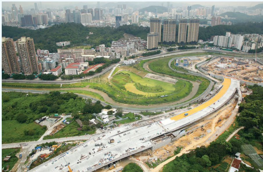
A flood retention lake built at the largest meander of Shenzhen River. The Shenzhen River can be seen on the outskirts of the retention lake on the right of the picture.
