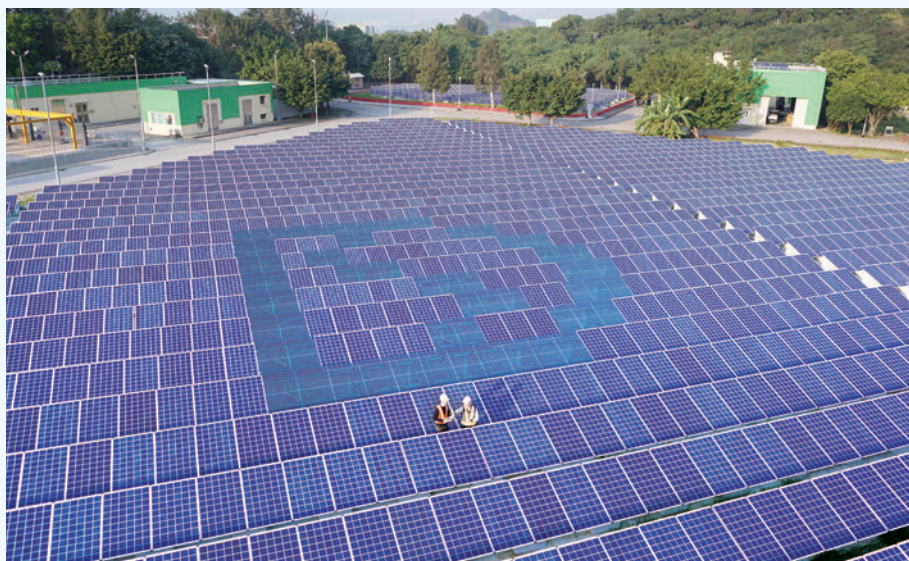
One of the three solar farm areas at the Siu Ho Wan Sewage Treatment Works
