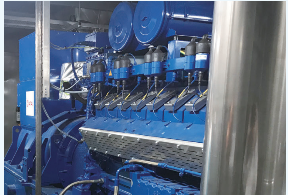
CHP generator at the Sha Tin Sewage Treatment Works
