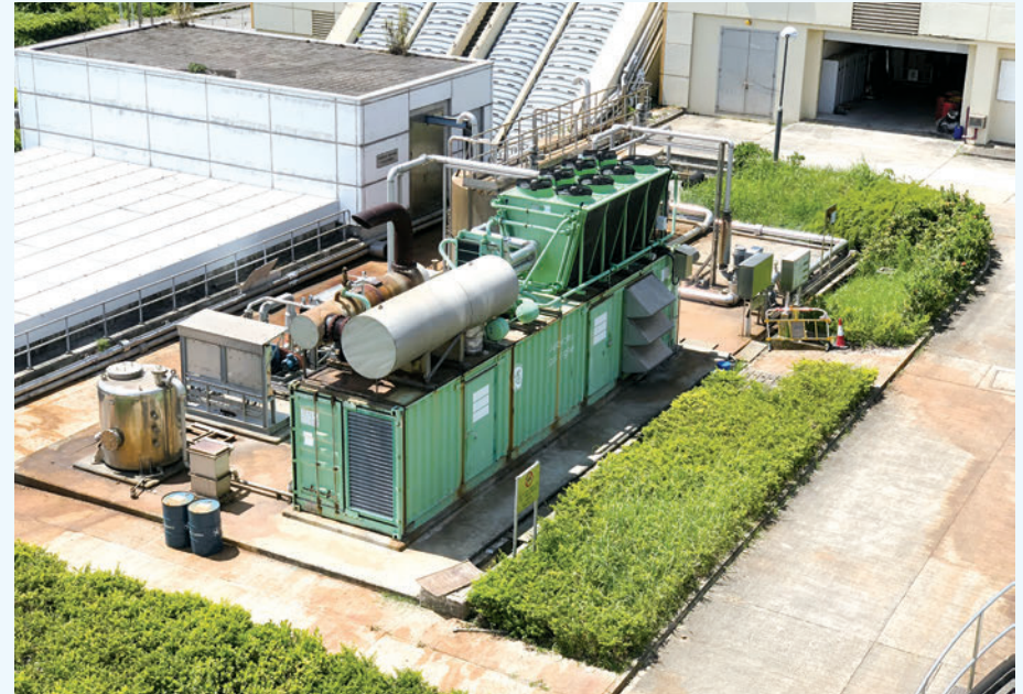
The Tai Po Sewage Treatment Works uses biogas as fuel to supply heat and electricity to the power generation system. These generators are large capital investments as each generator costs more than a few million dollars, depending on its capacity.
