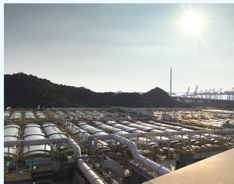
Sedimentation Tanks at the Stonecutters Island Sewage Treatment Works
