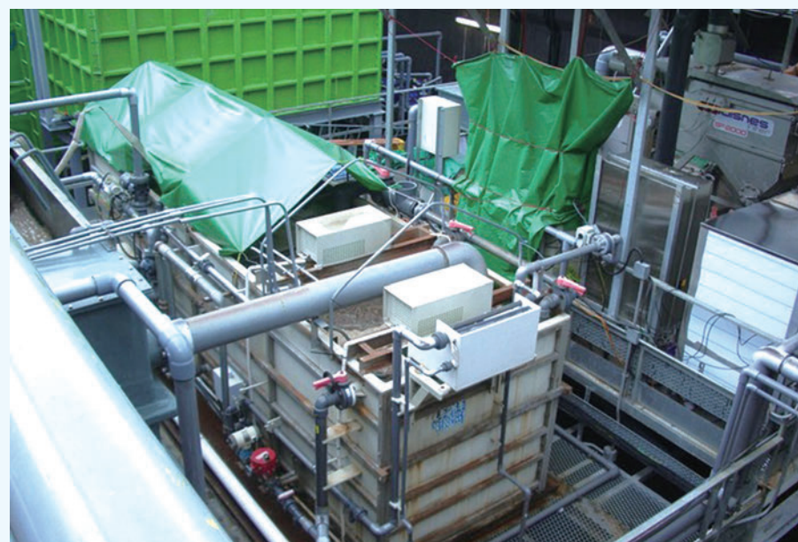
A pilot compact sewage treatment plant comprising a mechanical filter mesh and membrane bioreactors was set up at the Sha Tin Sewage Treatment Works to investigate their performances
