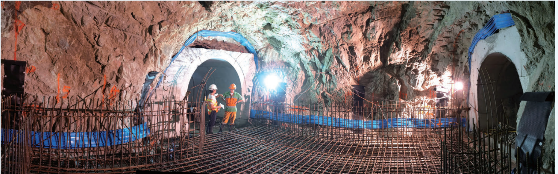
Excavation for the largest and longest drainage tunnel in Hong Kong amid hard rock stratum is much more than just a hole in the ground
