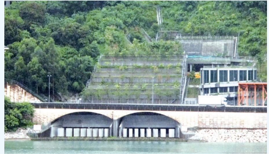
Buffer walls adjacent to the sea side of the outfall at Yau Kam Tau for modulating the speed of the collected stormwater to reduce the impact on seabed
