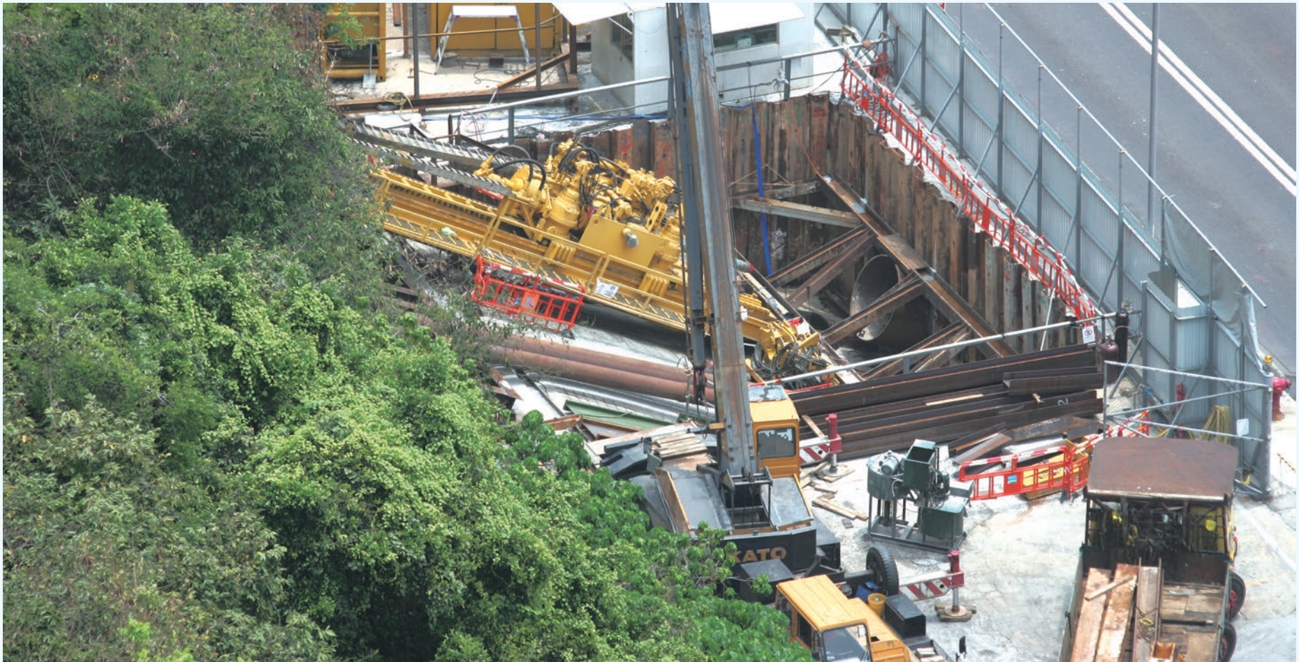
Horizontal directional drilling technology was employed for construction of the twin sewage tunnels between Ap Lei Chau (shown in the picture) and Aberdeen bypassing high voltage sub-marine electric cables
