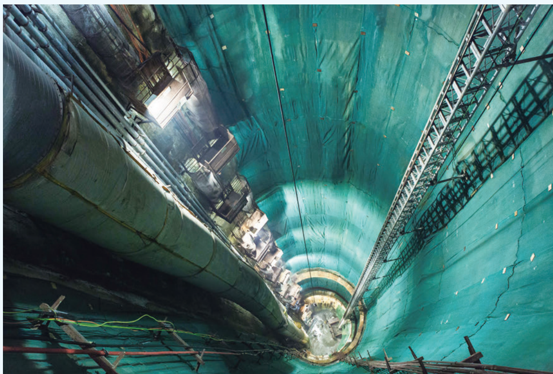
This drop shaft was used as an access during construction down to the world's deepest sewage tunnel
