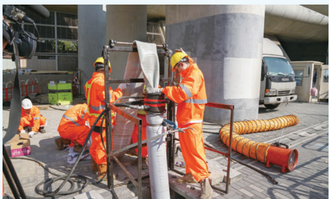
The liner is being pushed through a manhole into the underground pipe under repair
