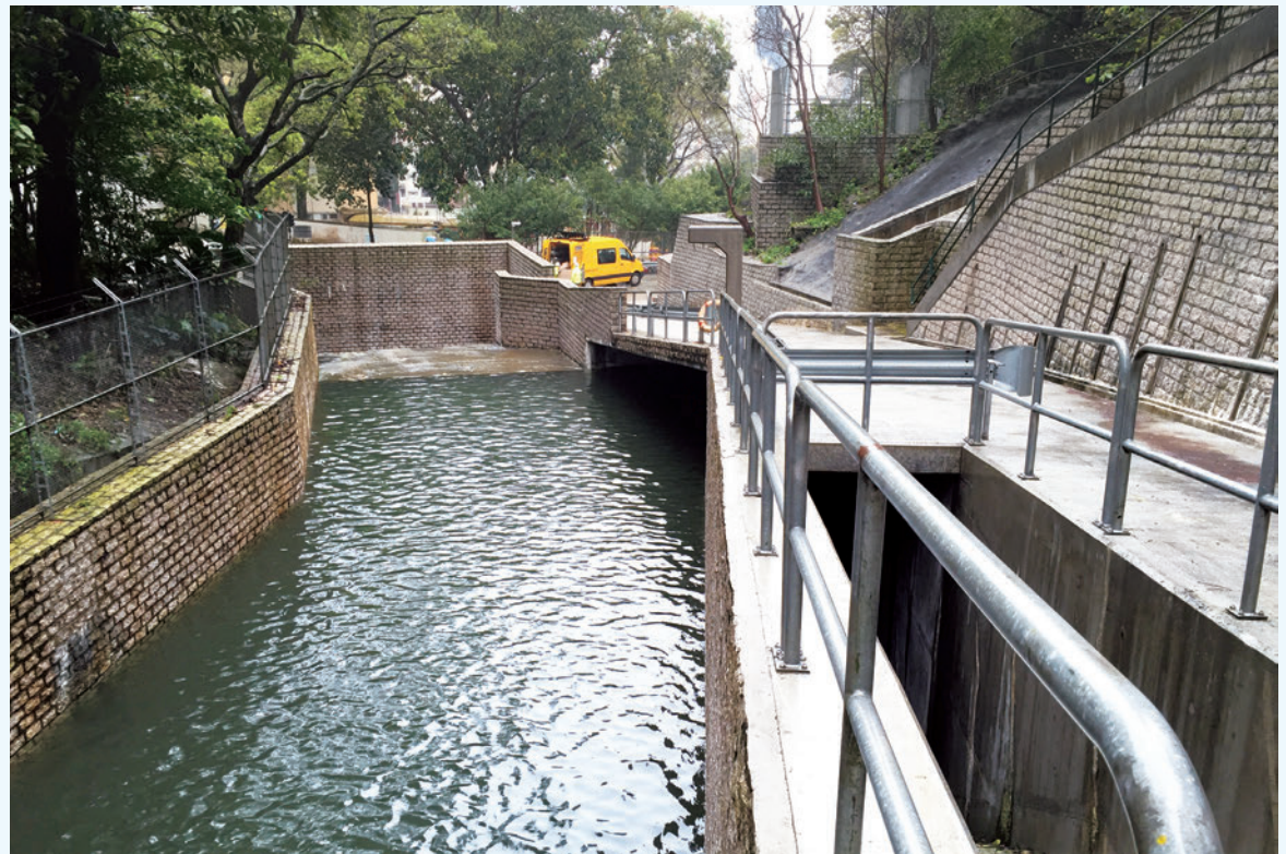
The intake at Tai Hang Road marks the eastern starting point of Hong Kong West Drainage Tunnel
