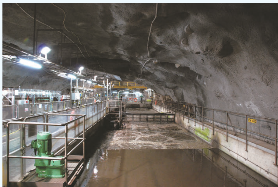
The two reactors in Stanley Sewage Treatment Works have combined Biofilm with Activated Sludge process
