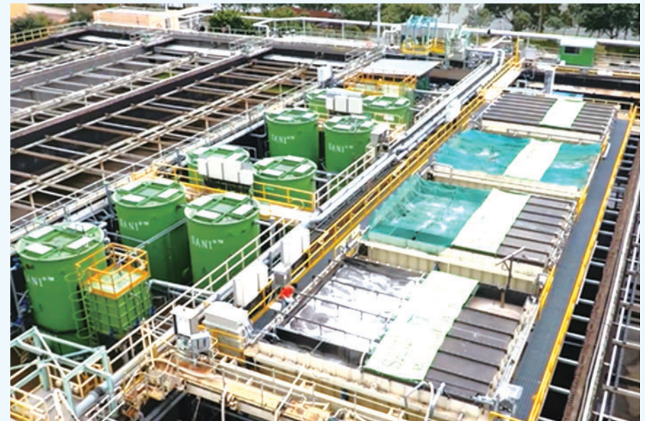
The SANI wastewater treatment technology was bestowed the Bronze Medal for Breakthroughs in Research and Development in the 2018 IWA Project Innovation Awards, and the Gold Award in the 2018 Hong Kong Green Innovations Awards
