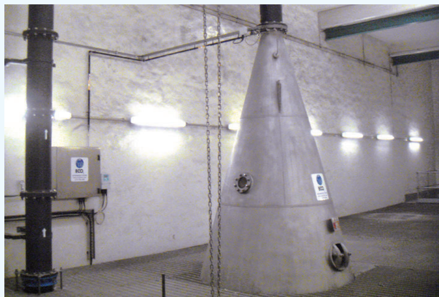
Part of the sewage will be conveyed to this conical oxygen dissolving tank where it is oxygenated and then returned to the main sewer
