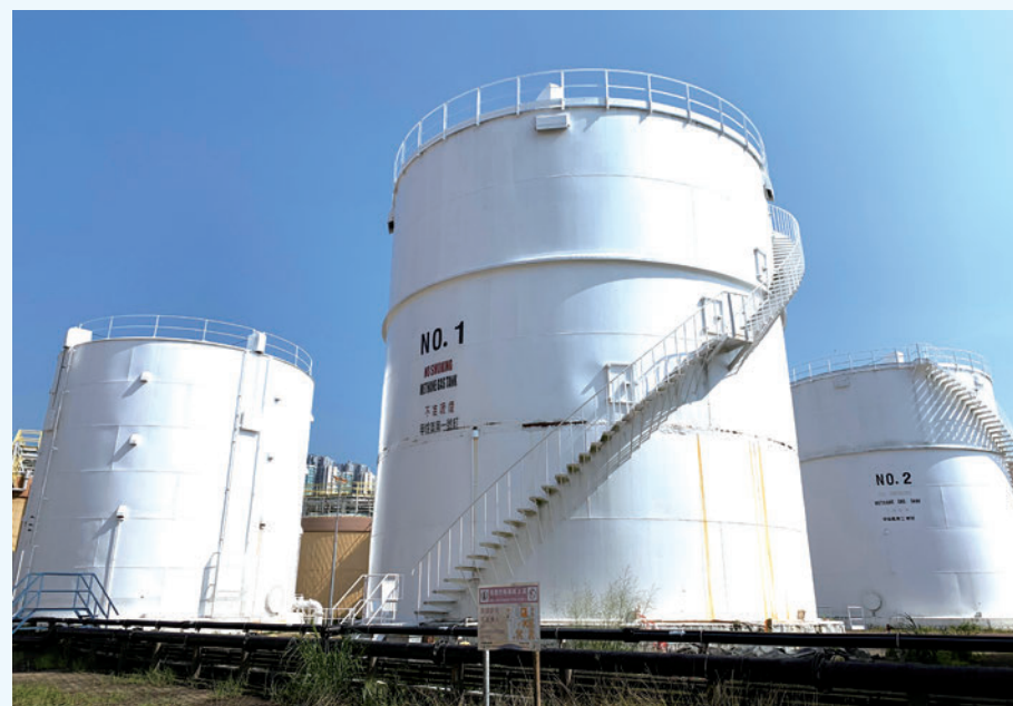
Biogas storage tanks at the Sha Tin Sewage Treatment Works
