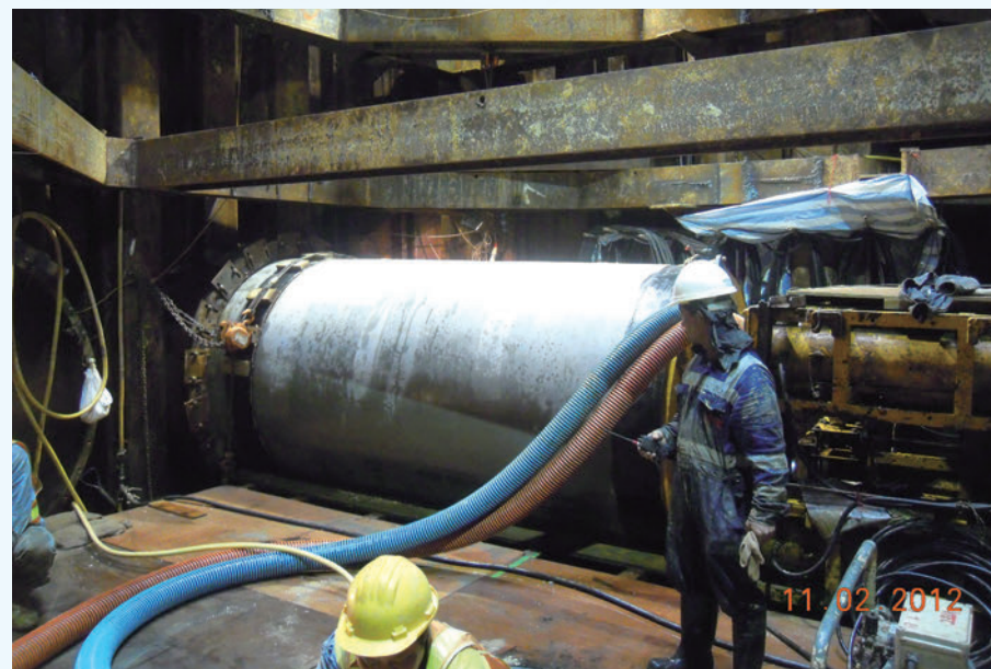
In recent years, the DSD has adopted the pipe jacking method to lay pipes across major obstacles, such as the Dongjiang watermains, railway lines and trunk roads.
