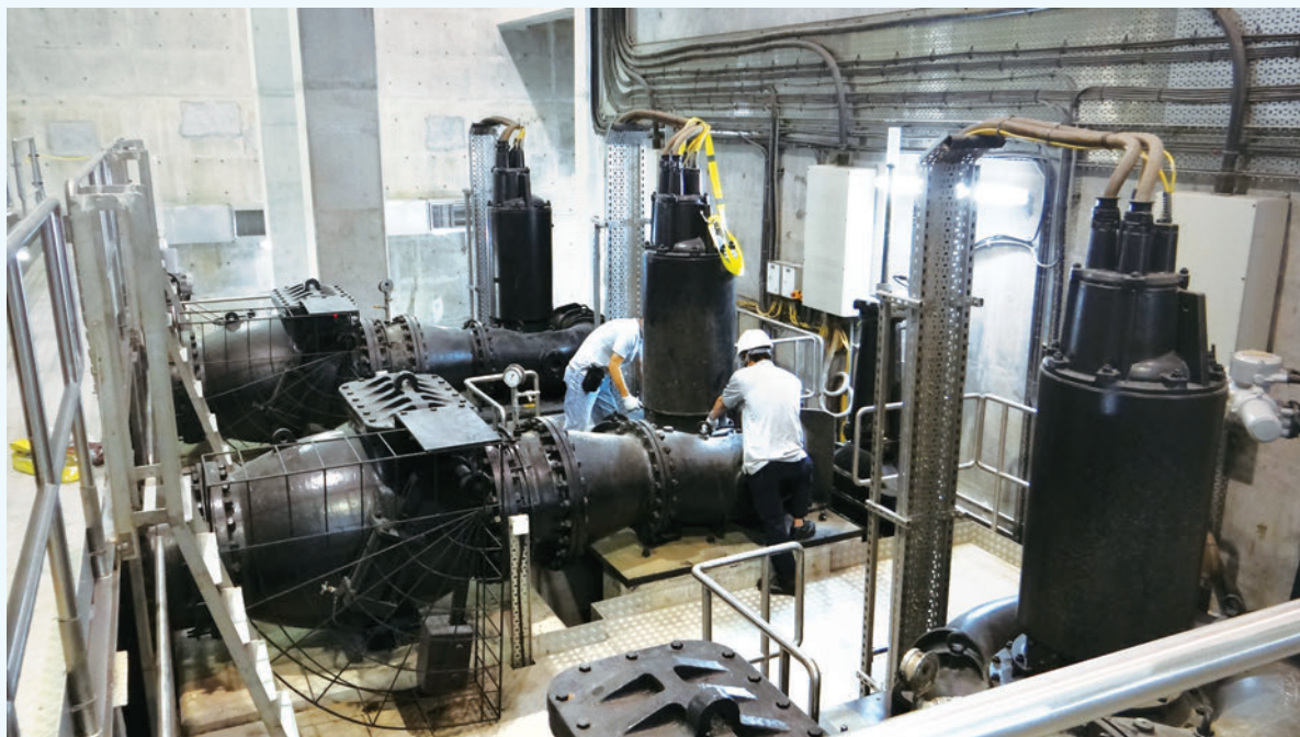
Maintenance of stormwater pumps in Tai Hang Tung Underground Stormwater Storage Scheme
