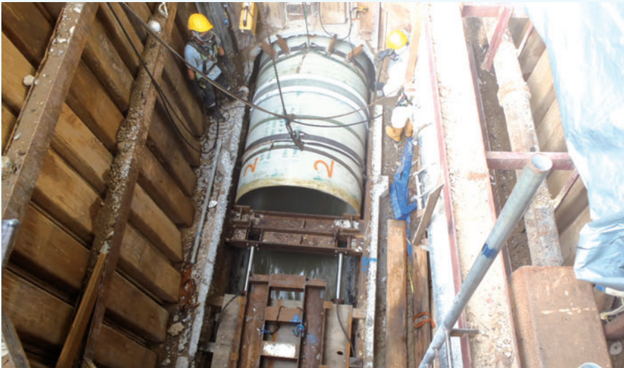
Hydraulic jack is used to push the fiberglass reinforced pipe into the underground pipe under repair
