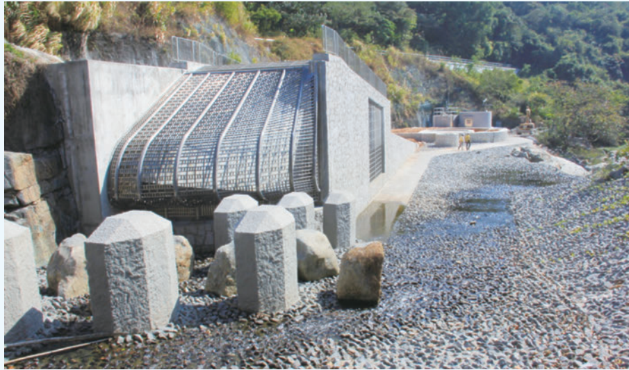
The intake at Tso Kung Tam was situated at a natural stream. Natural boulders and boulder-like concrete units were used to construct the buffers for blending with the natural environment.
