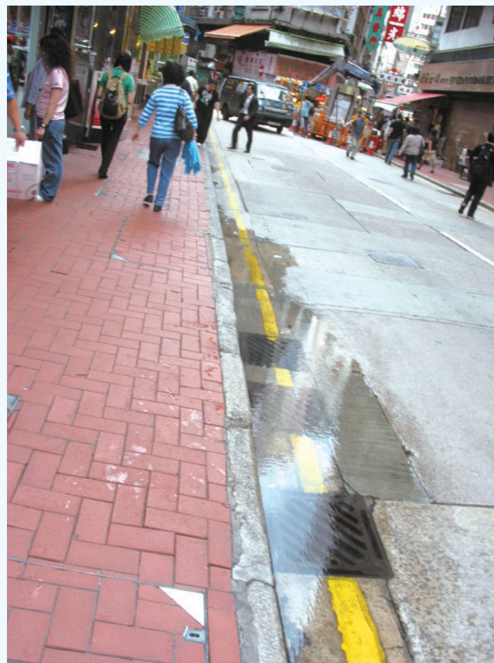
Wing Lok Street and Hillier Street junction at the lowest point of Sheung Wan flooded by seawater backflow during astronomical tides
