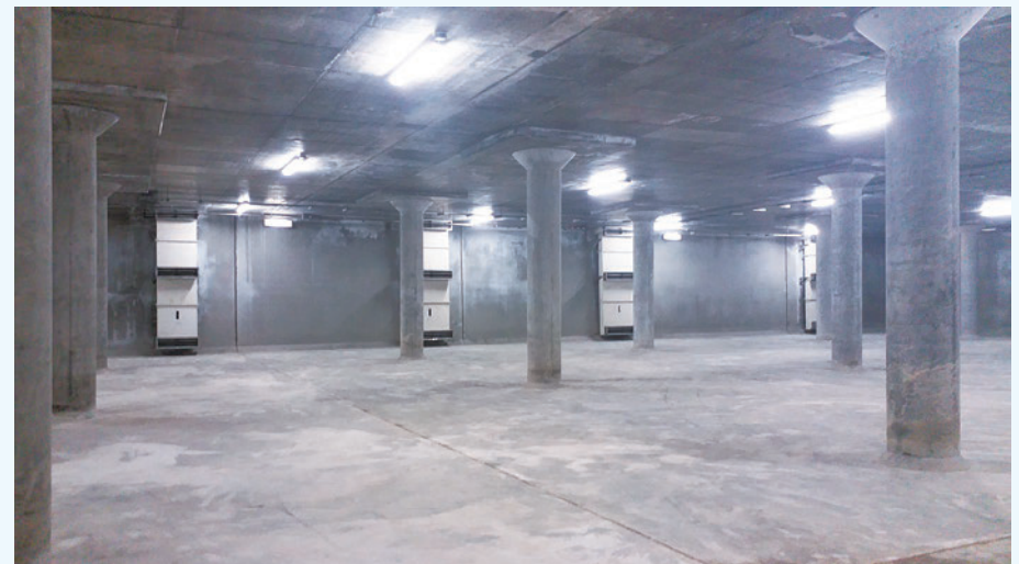
The On Sau Road Underground Stormwater Storage Scheme with a capacity of 18 000 cubic metres. Situated on a higher ground, the storage tank allows the stored stormwater to drain away by gravity without the need for pumping.
