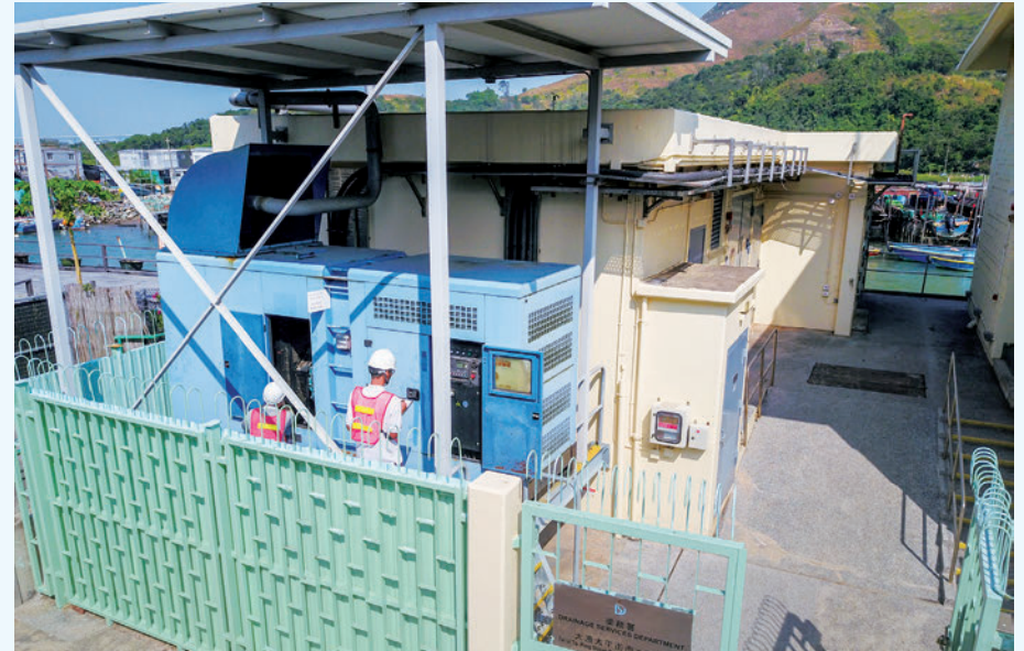
Monthly inspection of the emergency generator at the Tai O Tai Ping Street Stormwater Pumping Station
