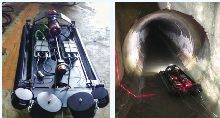
Remotely operated vehicle equipped with video camera, sonar and laser scanner for pipeline inspection.
