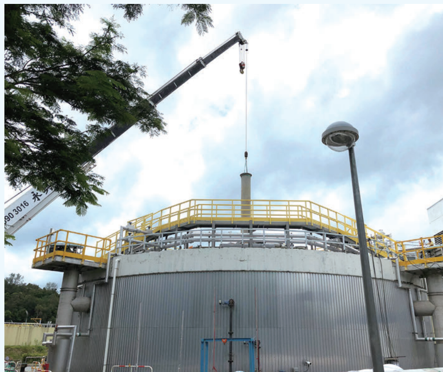
A section of draft tube is being installed in the sludge anaerobic digester at the Tai Po Sewage Treatment Works to facilitate the Food Waste/Sewage Sludge Anaerobic Co-digestion Trial Scheme
