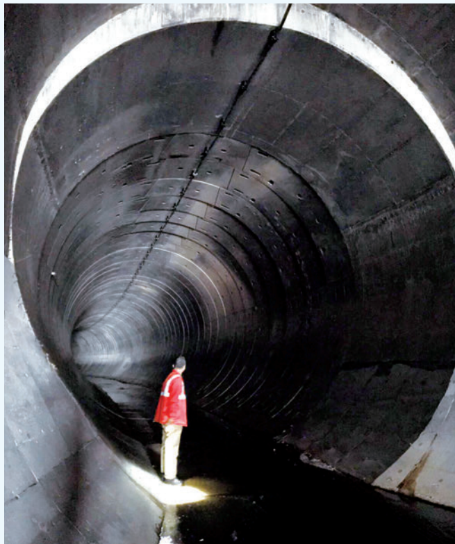
Hong Kong West Drainage Tunnel has a diameter varying from 6.25 to 7.25 metres, large enough to contain a 4.2 metres high double-decker bus.
