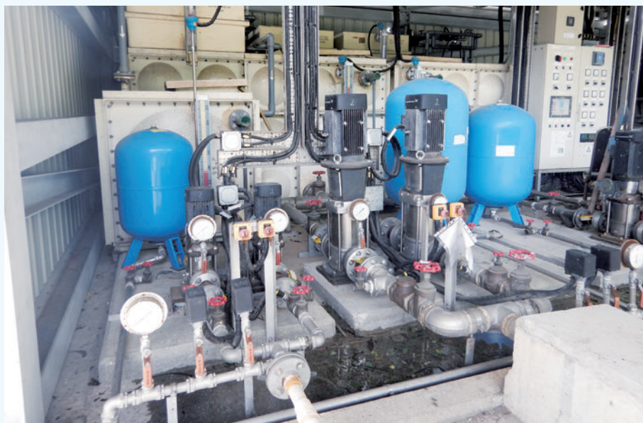
Water purification equipment for the Lai Chi Kok Drainage Tunnel stormwater harvesting system
