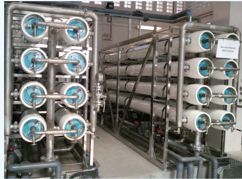
Reverse osmosis membrane components
