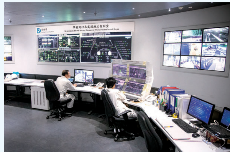
Main Control Room in the Main Pumping Station at Stonecutters Island Sewage Treatment Works
