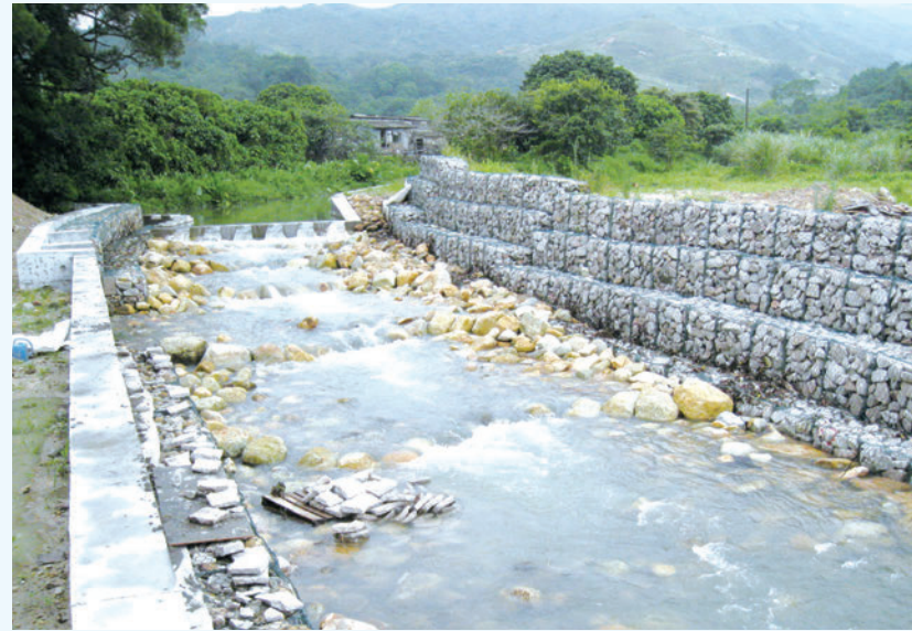
Fish ladders placed at the downstream of a concrete weir at the Pak Ngan Heung River in Mui Wo to help maintain ecological continuity between the upstream and downstream waters
