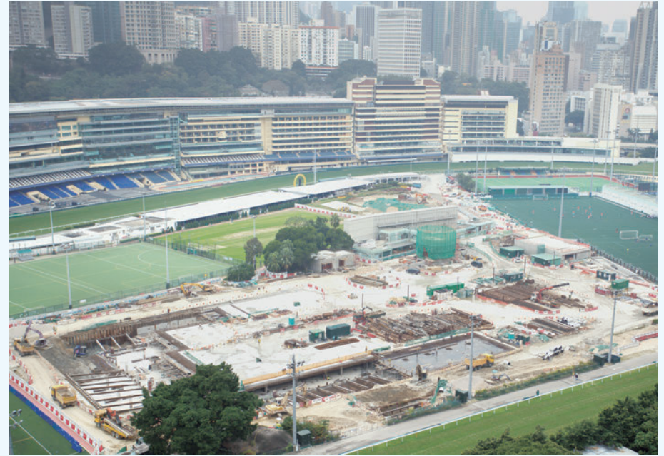
The HVUSSS was implemented in stages to achieve partial commissioning for early flood relief. Closure of the pitches in phases minimized disruptions to the public.
