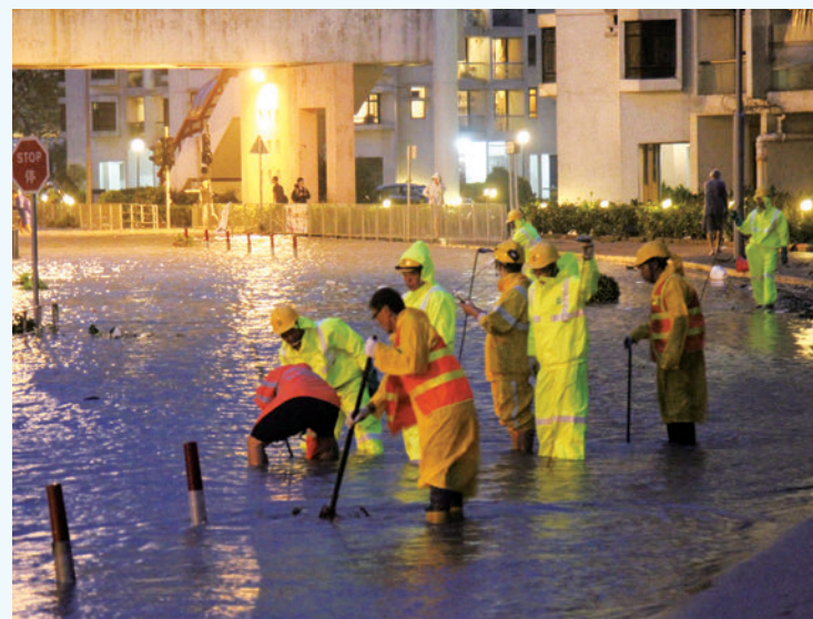
When Super Typhoon "Mangkhut" struck Hong Kong in 2018, the DLF helped clear up drainage blockages in flooded areas while the Hurricane Warning Signal No. 10 was in force.
