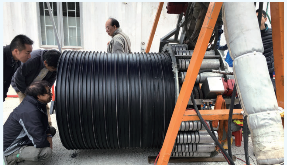
The project team is inspecting the spiral pipe liner wound by the winding machine
