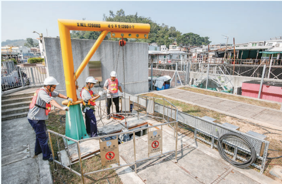
Inspection of stormwater pumping station in Tai O after passage of typhoon
