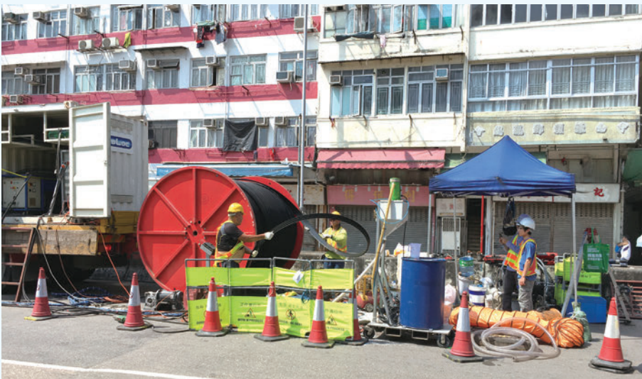
Steel-reinforced polyethylene strip is slowly wound by a winding machine and fed into the underground pipe from a manhole to form pipe lining
