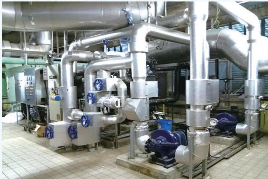
The CCHP tri-generation system installed at Sha Tin Sewage Treatment Works utilises the residual heat of generators to produce chilled water for cooling some facilities within the plant
