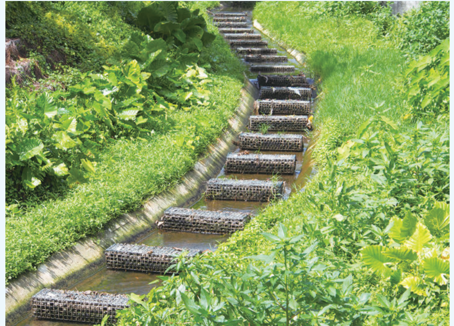
Cabions filled with bio-balls form biofilms for removing contaminants caused by livestock wastes
