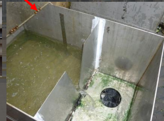
V-notch weir chamber
