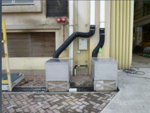
V-notch weir chamber (runoff measurement)
