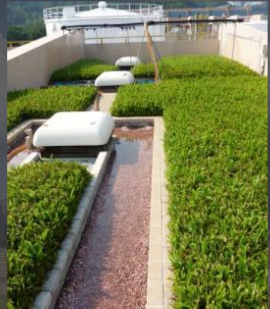
Water ponding in part of the roof (pebble path)
