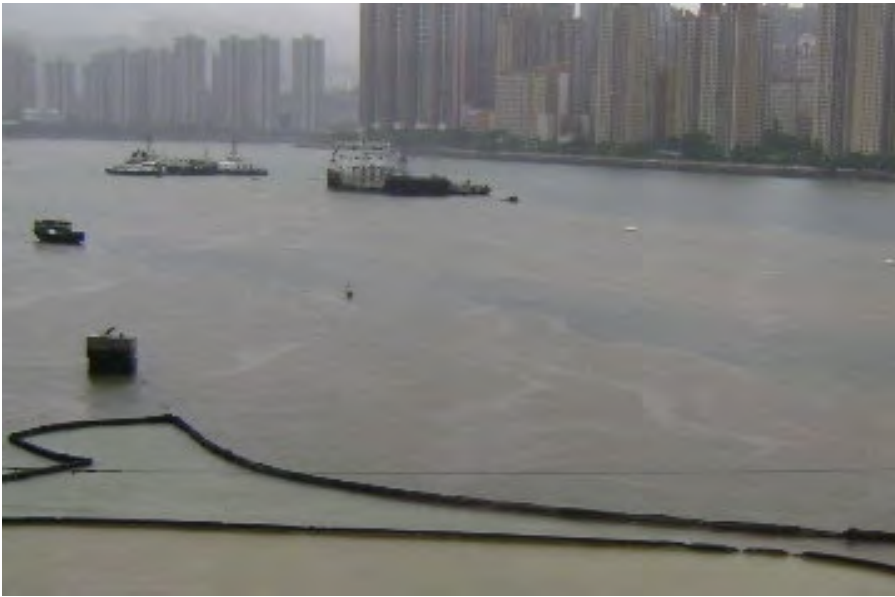
Site photo (The marine water between the inner and outer silt curtain was clearer than the marine water outside the construction site. No leakage of silt curtain was observed.)
