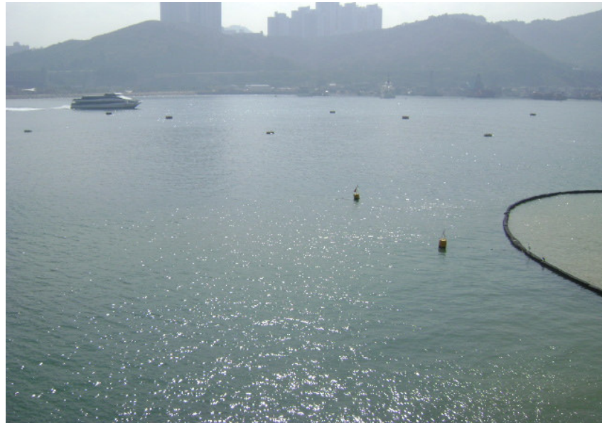
A photo showing slit curtain was functioning properly to prevent suspended solids dispersed away from the site
