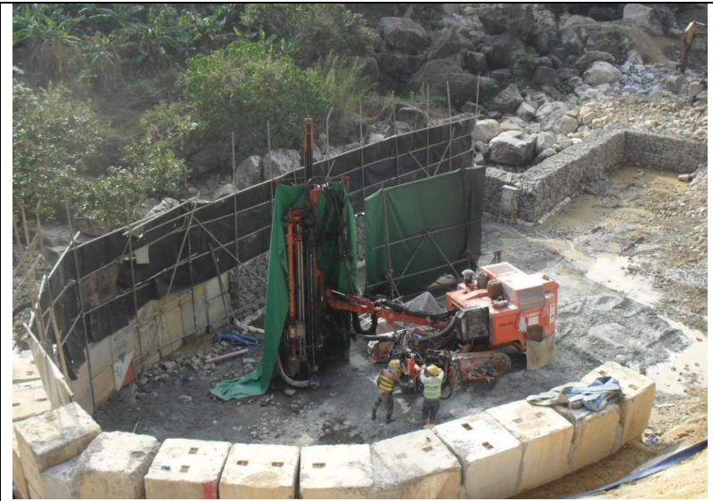
Sound insulation sheets were installed covering the working area during rock drilling in order to block the line of sight to the NSR.
