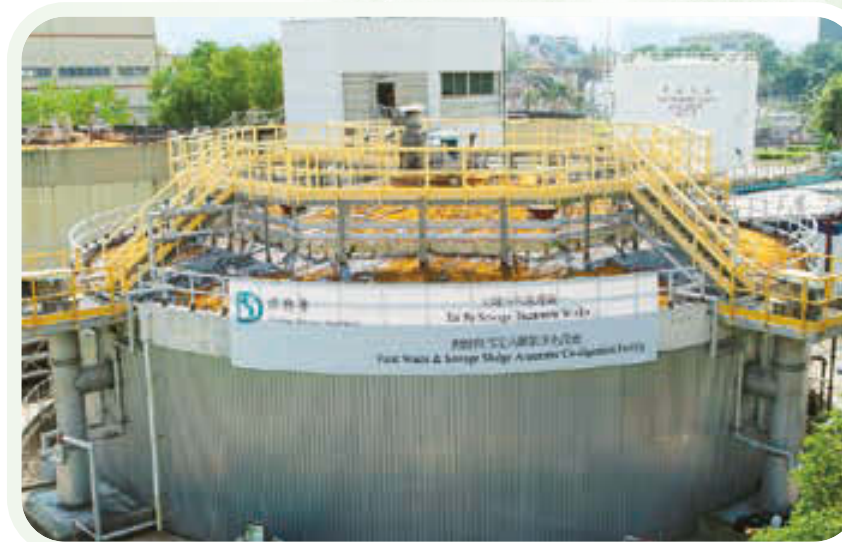
◀ 大埔污水處理廠內的廚餘、污泥共 厭氧消化設施 Food Waste and Sewage Sludge Anaerobic Co-Digestion Facility at Tai Po STW
