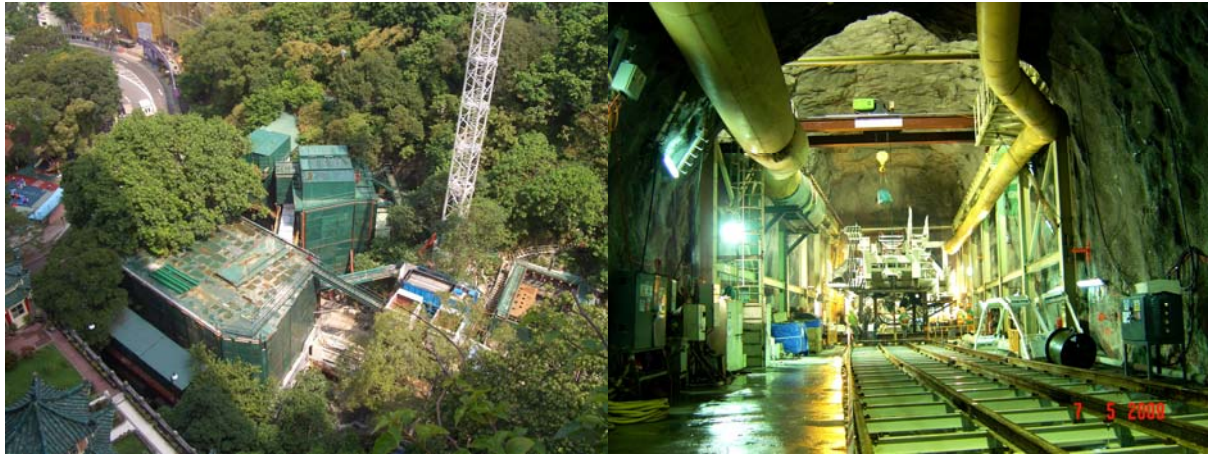
Figure 4 Eastern Portal TBM launch site bounded by busy public road, historic building and large secondary school (left); and Eastern Portal TBM launch chamber (right)
