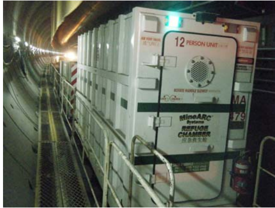
Figure 7 Refuge Chamber for tunnel workers during concurrent blasting
