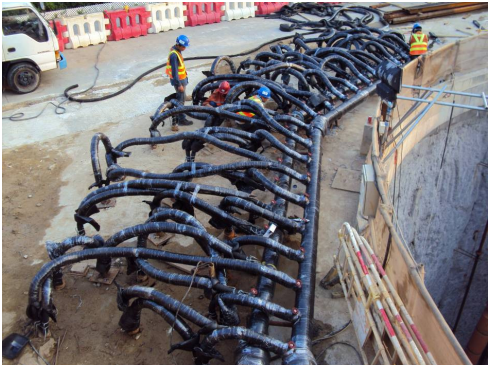
Photo 4 – Insulated Delivery and Return Pipes
