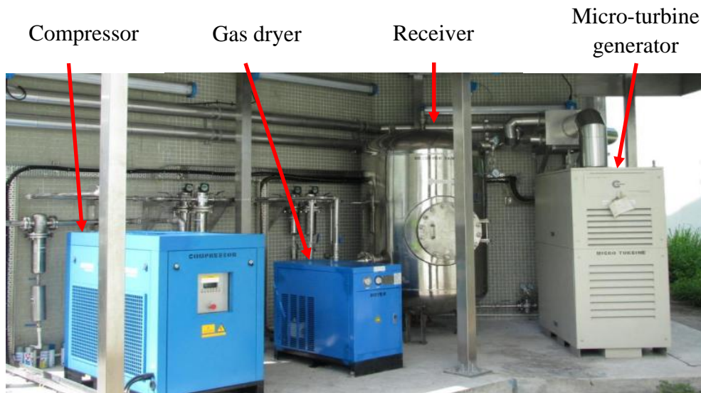
Figure 3: Micro-turbine generator system
