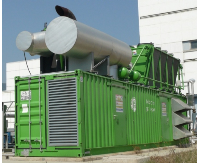
Figure 4: CHP installed in Tai Po Sewage Treatment Works
