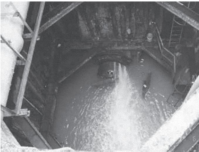
Figure 19 – Grout Plug Failure during TBM Breakthrough
