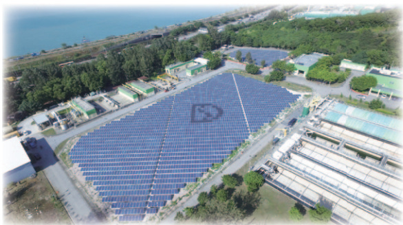
Solar farm at Siu Ho Wan Sewage Treatment Works
