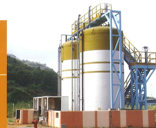
三氯化鐵儲存缸 Ferric Chloride Storage Tanks
