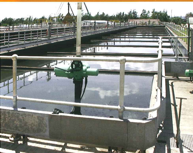
沉澱池 Sedimentation Tanks
