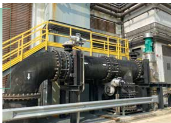
昂船洲污水處理廠的水力發電系統 Hydro-turbine system at Stonecutters Island Sewage Treatment Works
