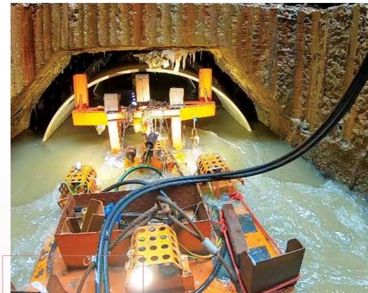
應用遙控機械人於運作中的 污水幹渠內鋪設喉管 Deploying robotic machine for lining installation works in existing box culvert with live sewage flow
