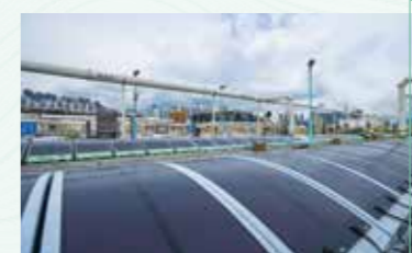
昂船洲污水處理廠內弧形沉澱池蓋上的柔韌薄膜太陽能光伏系統 Flexible thin-film PV system on curved sedimentation tank covers in Stonecutters Island Sewage Treatment Works
