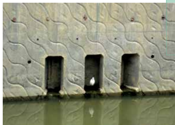
河岸牆洞 Holes in river walls
