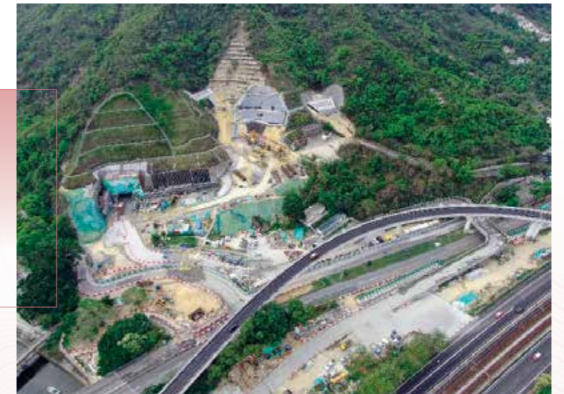
「搬遷沙田污水處理廠往岩洞」第一階段建造工程 Stage 1 works of “Relocation of Sha Tin Sewage Treatment Works to Caverns”
