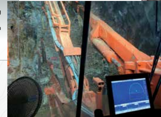
珍寶操作員於操控室內監察鑽挖工程 Monitoring drilling operation by a Jumbo operator in the control room
