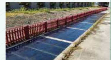
小蠔灣污水處理廠的可踏式太陽能光伏板 Steppable PV panels in Siu Ho Wan Sewage Treatment Works
