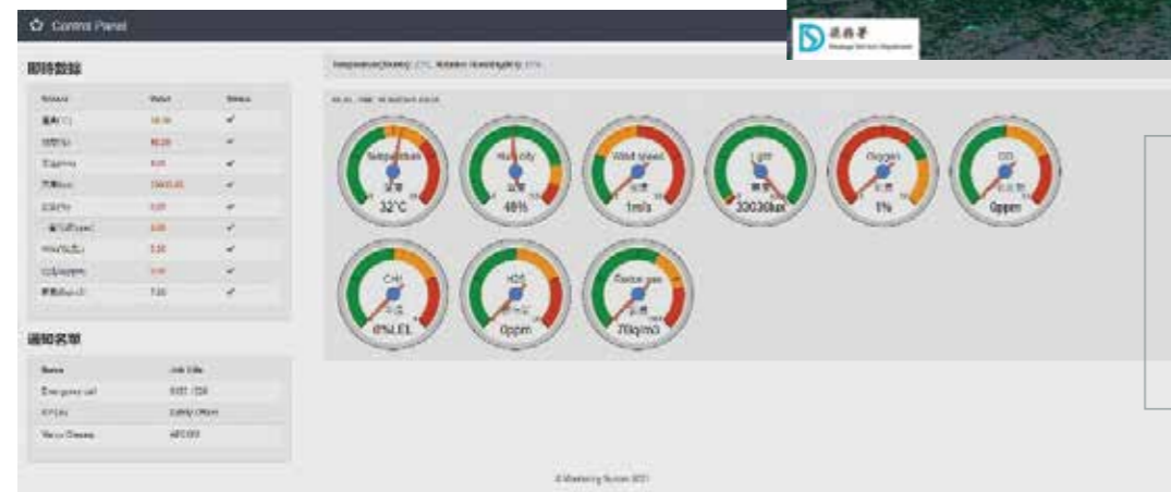
透過系統實時監測隧道內的各類氣體 Monitoring in real time through the system various types of gas in the tunnel
