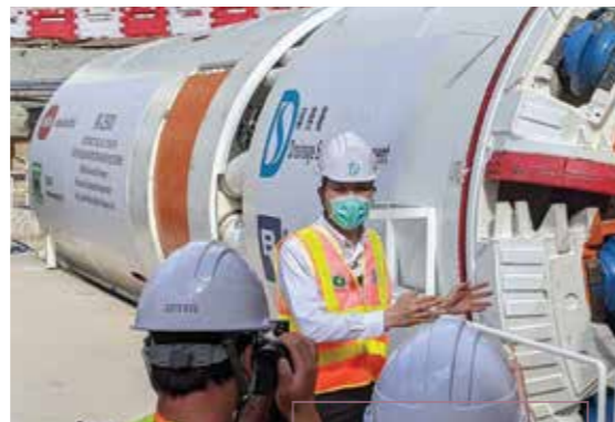
工程師葉浩朋先生向記者介紹隧道鑽挖機的組裝過程 Engineer, Mr Raymond IP Ho-pang presented the assemble process of the tunnel boring machine
