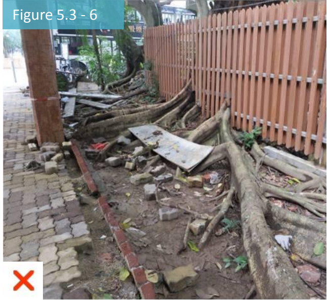
Fig. 5.3 - 6 Tree species with vigorous root systems (such as Ficus spp. , Delonix regia , etc.) should not be planted at the boundary edge/narrow planter/pit as their roots may twist and become unstable, or cause pavement uplifts or damage to the adjacent property.
