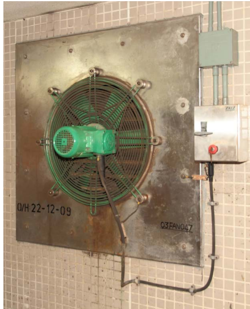
Photo 2: Wall-mounted Ventilation Fan (9 nos.)
