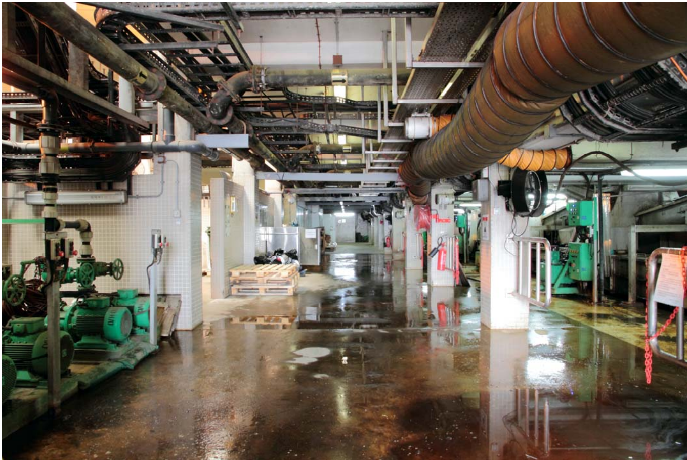
Photo 1: Sludge Dewatering House Equipment Hall (View A)
